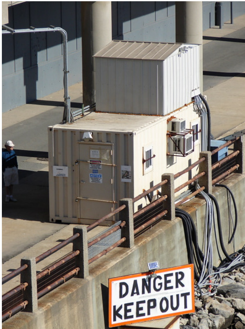
Photo 4.3.8.1-2. Verdant Power's control room and associated equipment at the RITE Demonstration Site.
